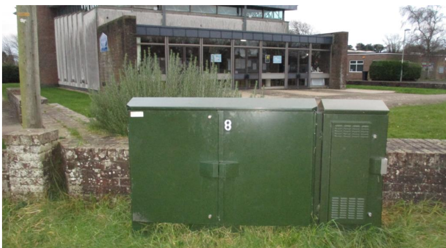
Cabinet in position (in front of church).
